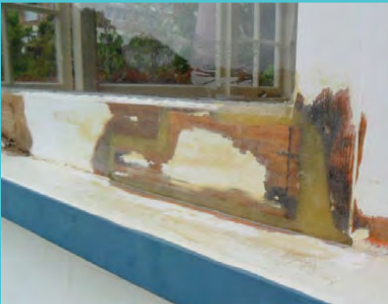
WITH THE USE OF EPOXIES, DETERIORATED SECTIONS OF WOOD CAN BE SCRAPED OUT AND INFILLED. SINCE MOST WOOD IS PAINTED, REPAIRS LIKE THIS ARE CONCEALED AND CAN LOOK AS GOOD AS NEW.
