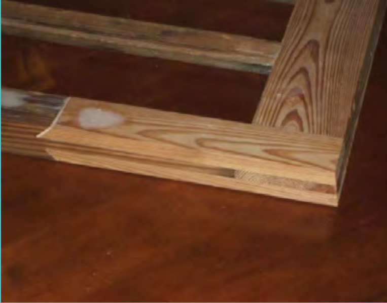
BADLY DETERIORATED SECTIONS OF WOOD CAN BE REMOVED AND A NEW PIECE (CALLED A DUTCHMAN) CAN BE INSTALLED.
